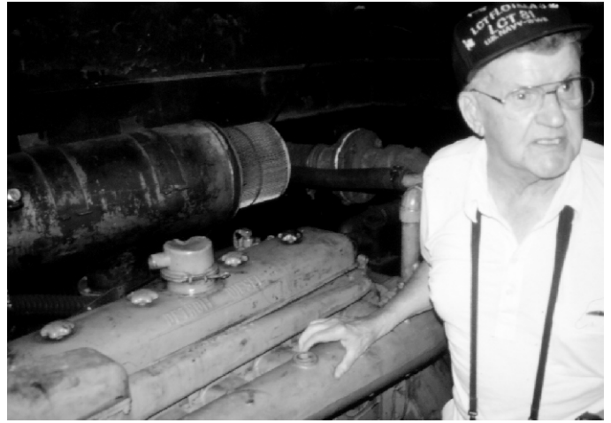
Doug Swanson inspects the original Gray Marine Diesel engines below decks where he spent time as electrician's mate on the LCT-81.
